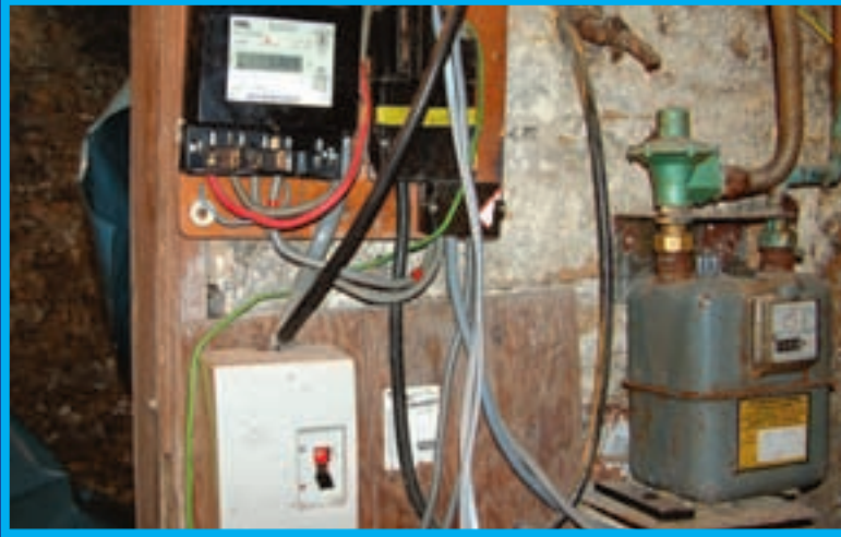
Cannabis cultivators can cause fires in properties by tampering with wiring
